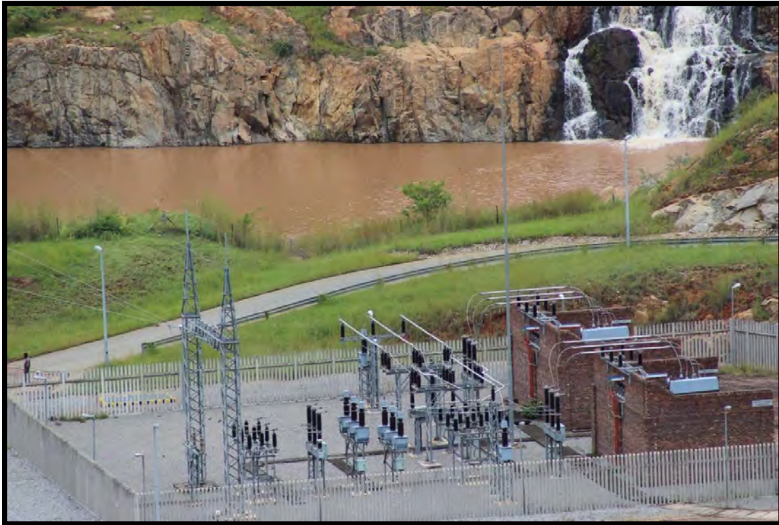
FIGURE 2 - MAGUGA DAM HYDRO POWER PLANT IN THE KOMATI RIVER
